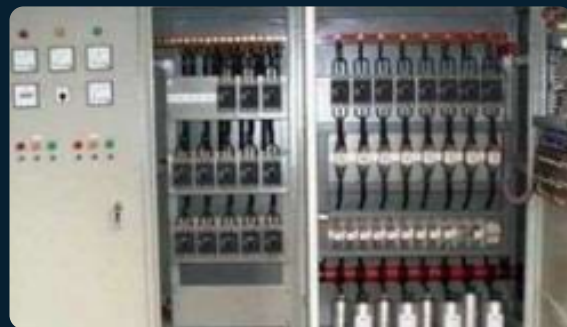
Panel Capacitor Bank
