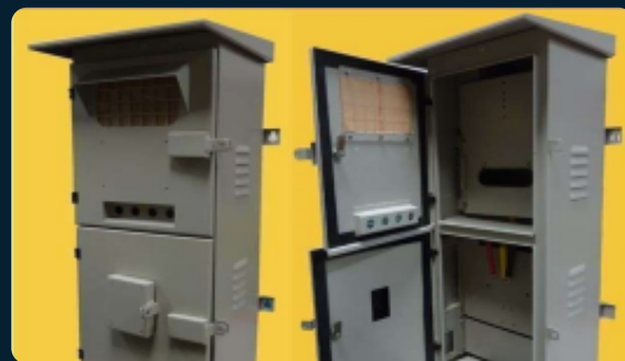
Panel Kwh Meter
